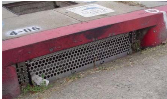
Retrofitted catch basin to prevent trash from entering the storm drainage system.
