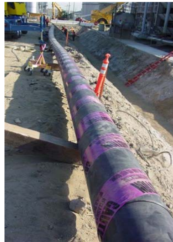
Purple pipe networks help expand recycled water distribution
